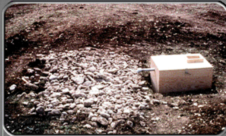
Baffle grease trap
