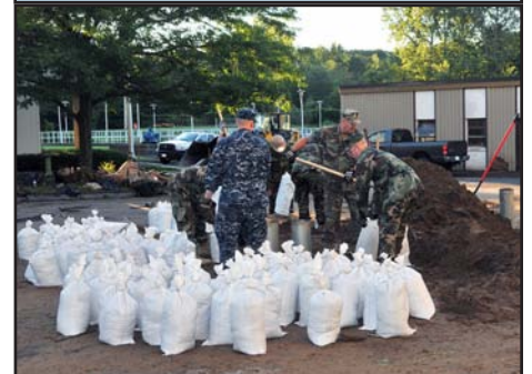
Sandbagging doesn't get easier with age. New York Naval Militiamen team together to fill each sandbag by hand so that another team can place them around the Schenectady sewage treatment plant. Photo by Senior Master Sgt. Willie Gizara, 109th Airlift Wing.
