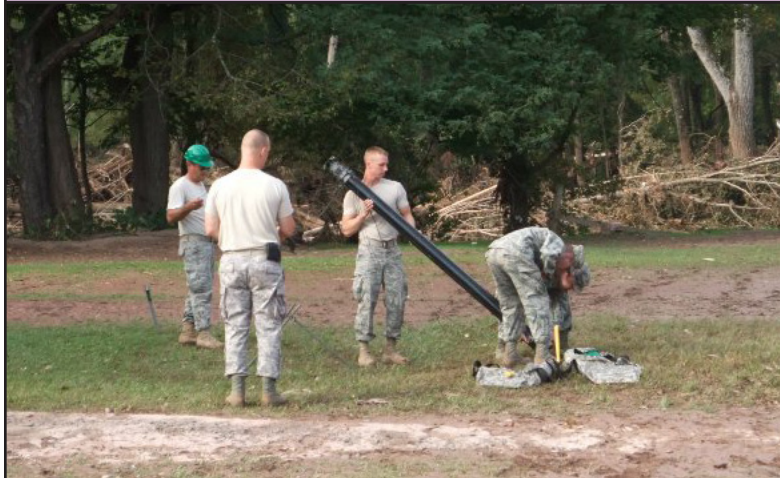
New York Air National Guard Airmen of the 174th Fighter Wing JISCC Team install an antenna mount near the Emergency Operations Center in Prattsville to provide a communications infrastructure to first responders and flood victims in the area following the devastating floods following Hurricane Irene.
