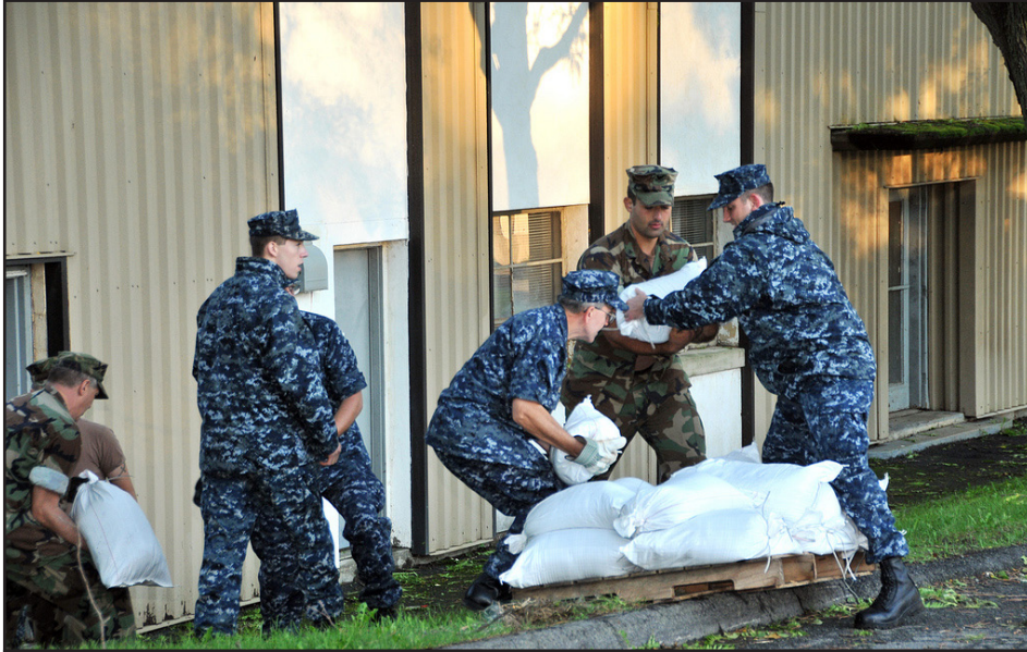
New York Naval Militia members assist in erecting a sandbag wall around the Schenectady sewage treatment plant to prevent flooding from the Mohawk River Monday, Aug. 28. Hurricane Irene swept through New York leaving many areas devastated by flood. Photo by Senior Master Sgt. Willie Gizara, 109th Airlift Wing.
