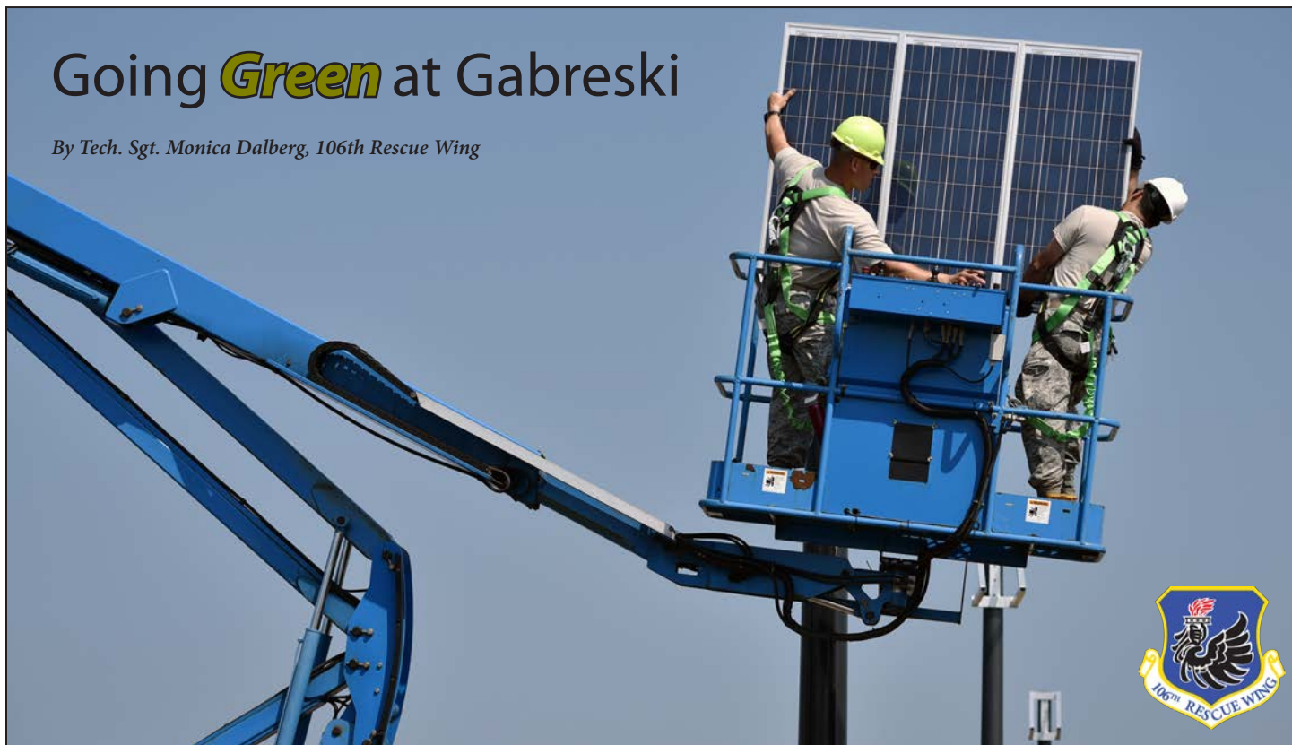
Staff Sgts. Edwin Laporte and Hector Gomez, members of the 106th Civil Engineering Squadron, 106th Rescue Wing install a solar panel at F.S. Gabreski Air National Guard airport Sept. 8. The solar panels program is part of a larger plan to reduce energy usage and save money by investing in renewable energy sources on base. Photo by Staff Sgt. Christopher Muncy, 106th Rescue Wing.
