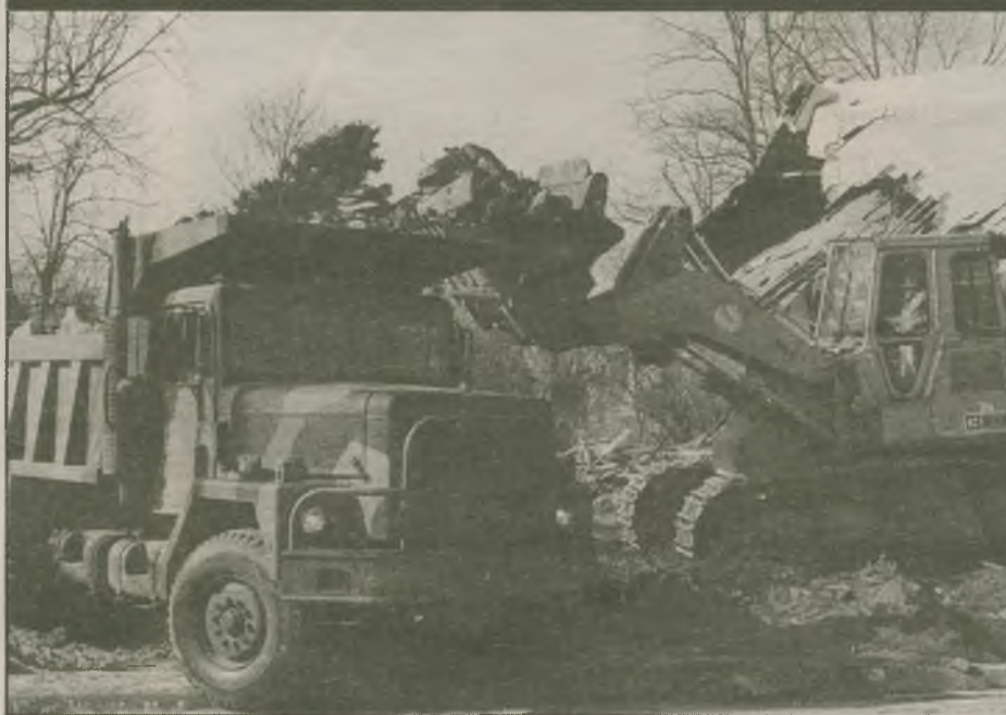
A 5-ton Dump Truck of the 204 th Engineer Battalion is filled with demolition debris by a civilian contractor working for the Long Island community of Bayshore. The New York National Guard Counterdrug Program in conjunction with the 204 th is helping the community get rid of abandoned buildings that drug dealers had been using. New low-income housing construction is planned once the old buildings are gone. Look for the story in the March-April issue of Guard Times. Photo courtesy of the 204 th Engineers.
