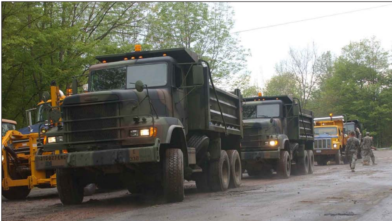
Dump trucks from the 204 th Engineer Battalion and the 827 th Engineer Company of the New York Army National Guard partner with trucks from the NYS Dept. of Transportation, NYS Dept. of Environmental Conservation and Towns of Hancock and Colchester to haul dirt to the areas washed away in mid-June by flash floods along the Holiday Brook in the two Adirondack communities.
