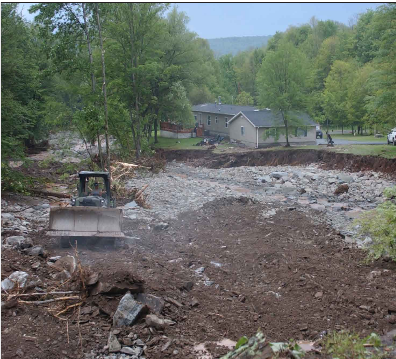
Spc. Patrick E. McCarthy, 827 th Engineer Company, New York Army National Guard, operates a D7 bulldozer in an attempt to restore the washed away portions of the Holiday Brook Road and return the Holiday Brook back to its original course. A flash flood eroded portions of the road and damaged several homes, destroying one. Four persons were reported missing after the flood waters receded.
