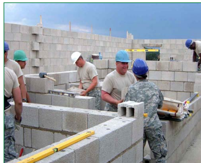
Specialist Edward Flanagan hands off a concrete block to Pfc. Popi Begum during the construction of the interior walls at the MOUT building. Hard at work in the background are Spc. Micah Wycoff, Spc. Brandon Sklar and Staff Sgt. Paul Moodie. Photo courtesy of 1156 th Engineer Company.
