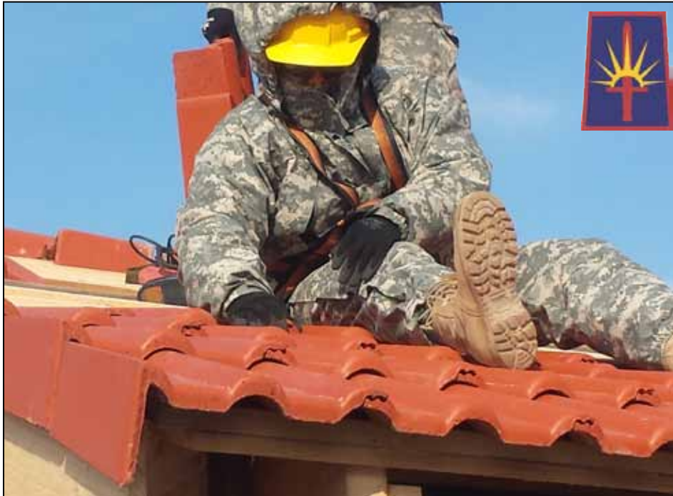
Pfc. Dillon Smith, 1156th Engineer Company, installs European roofing tiles on a building at the Joint Multinational Readiness Center, Hohenfels, Germany, in March. Along with other accomplishments, company troops and two New York Air National Guardsmen constructed two multi-use buildings, complete with wiring during a three-week period. Photo by Capt. Dan Colomb, 1156th Engineer Company.
