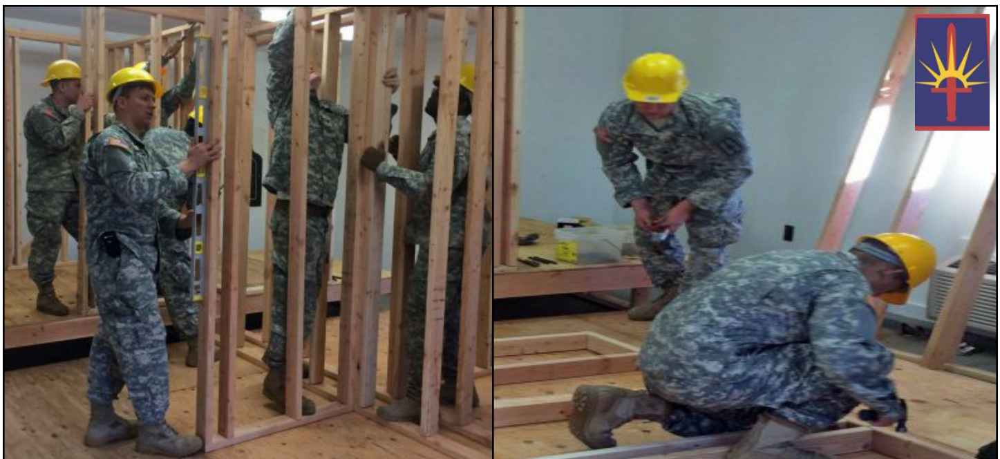
Soldiers of the New York Army National Guard's 1156th Engineer Company practice their skills by constructing walls — complete with wiring and plumbing fixtures — in Building 95 on March 3. Photo courtesy of 1156th Engineer Company.
