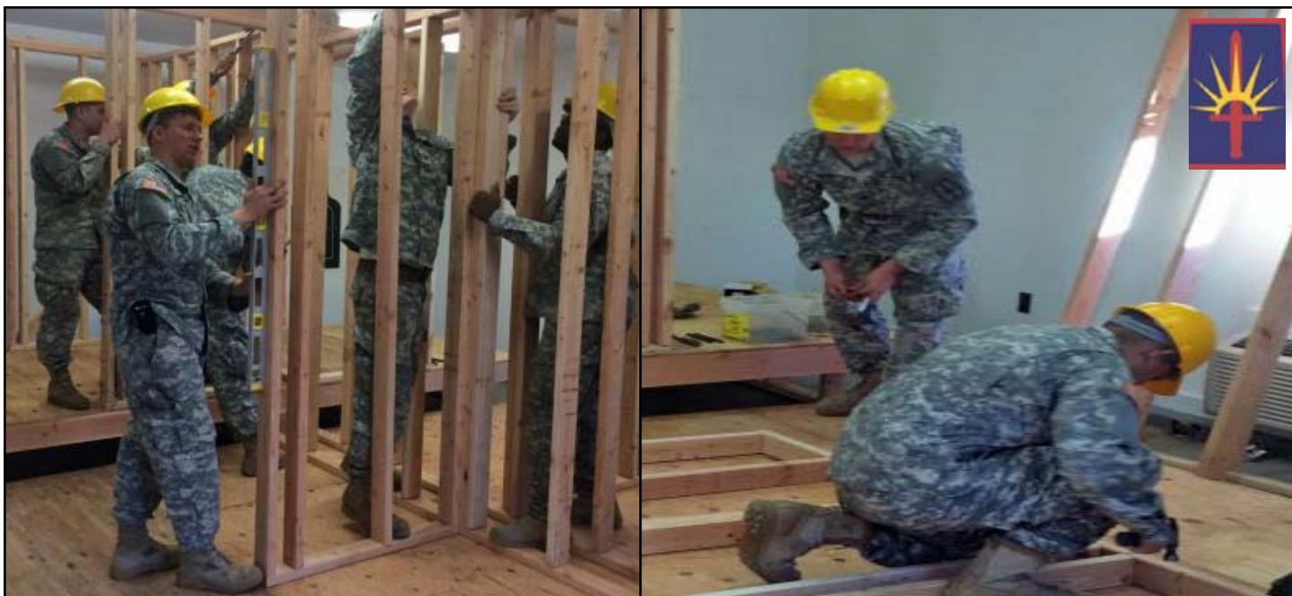
Soldiers of the New York Army National Guard's 1156th Engineer Company practice their skills by constructing walls — complete with wiring and plumbing fixtures — in Building 95 on March 3. Photo courtesy of 1156th Engineer Company.
