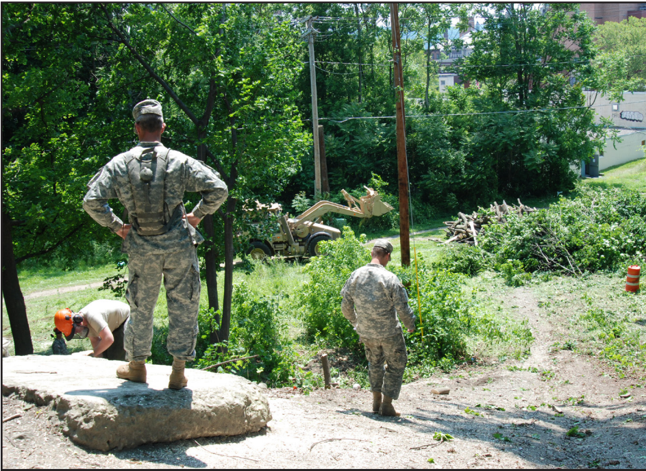
Sgt. Danny Edwards of the 152nd Engineer Company from Buffalo watches Soldiers as they clear fallen trees and prepare to cut another as part of the Erie Canal clean up project. Photo by Sgt. 1st Class Steven Petibone, Guard Times Staff.
