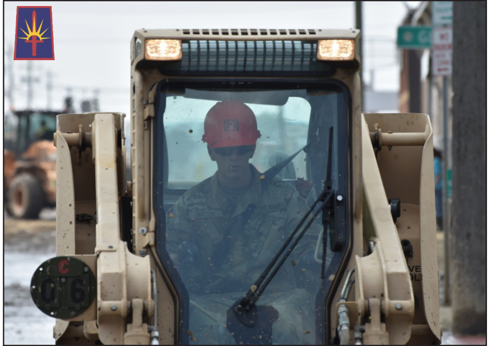
Pfc Dakota Button, assigned to the 827th Engineer Company clears flooding mud and debris in Binghamton, N.Y., Aug. 15, 2018. Soldiers were responding to flooding throughout many areas of Binghamton assisting civilians and the Department of Transportation. Photo by Spc. Andrew Valenza, Joint Force Headquarters.
