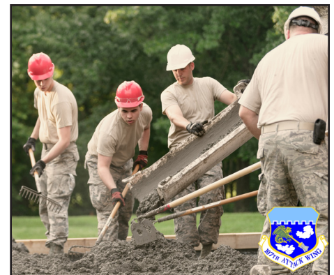
107th Civil Engineer Squadron Airmen pour concrete to create a ramp at the West Virginia School for the Blind and Deaf in Romney, W. Va., June 21, 2018.
