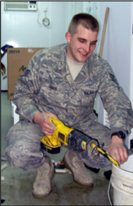
Staff Sergeant David Loder, 107th ARW, cuts a pipe for a hot water tank installation, Jan. 30, at Sather Air Base, Iraq. Photo by Senior Airman Peter Dean.
