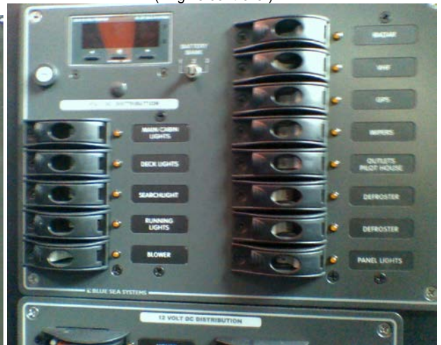
(Electrical breaker panel)
