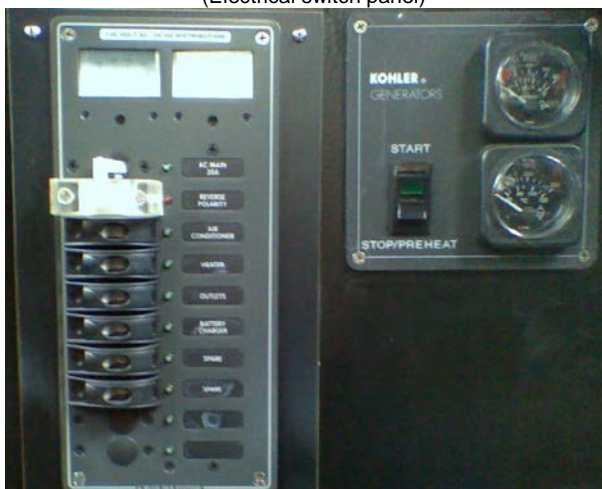
(Electric control and genset panel)
