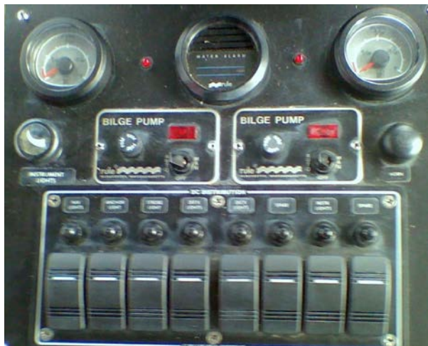
(Electrical switch panel)
