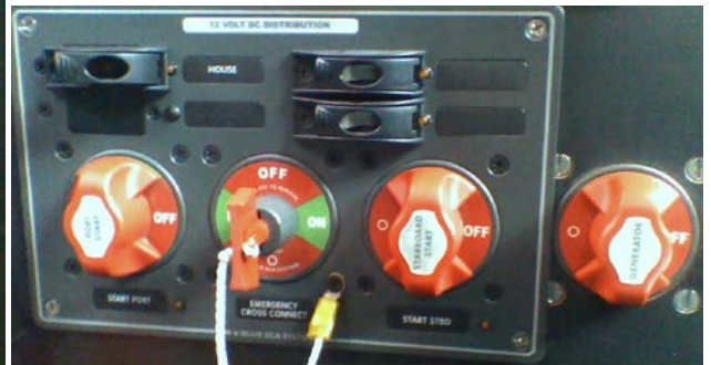
(Battery isolator switches)
